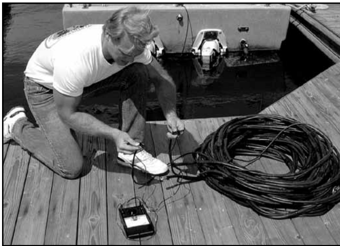
Figure 7 Preliminary testing of the umbilical with a volt-ohm meter to check for continuity.
